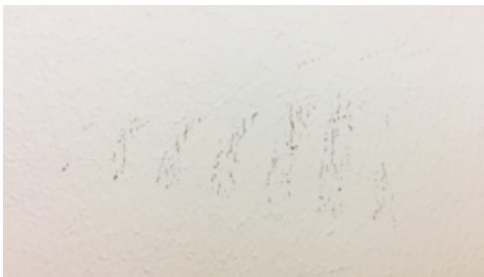
Figure 2: Example of scuffing on a standard wall paint [2].
